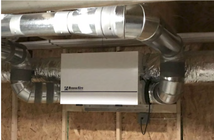
Typical HRV installed in a Unity Home
