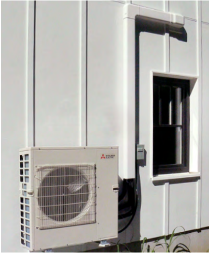
wall-mounted compressor and refrigerant lines
