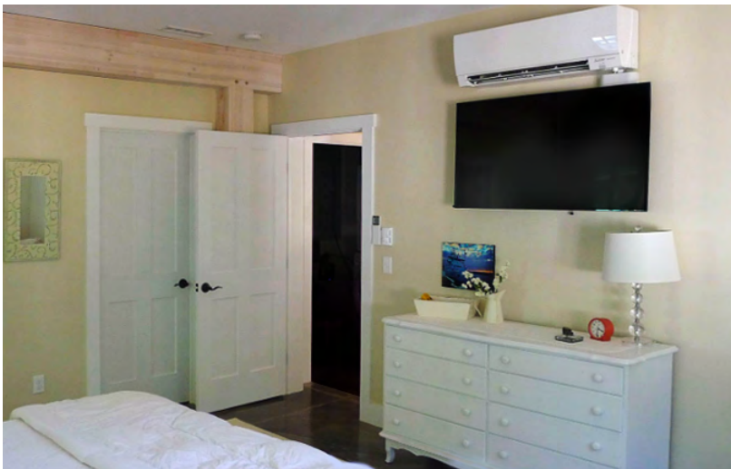
wall cassette in bedroom supplying fresh air
